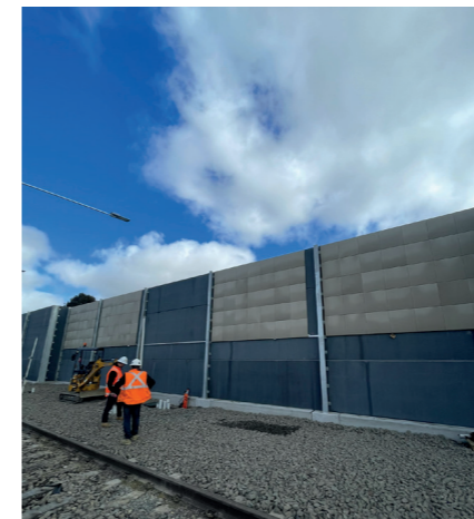
Noise barrier constructed along rail line on Lackeys Road measuring 250m in length and 5.5m high. View from rail corridor.
