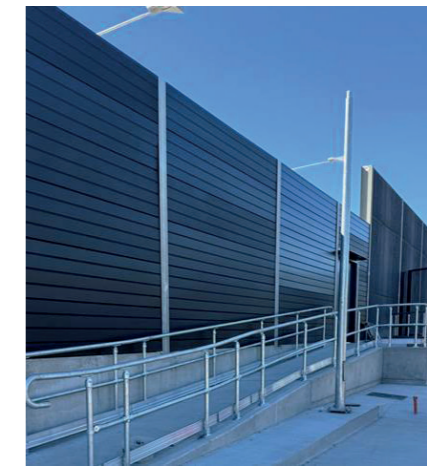
Acoustic wall upgrades replaced sections of the concrete wall with sound-absorbing aluminium-clad composite panels featuring a recycled PET core.
