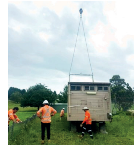
Shed donated to Moss Vale High School for use by their Sports Department
